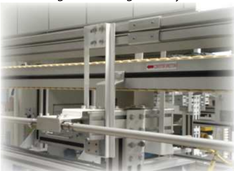
Automated side guide installed at straight section
